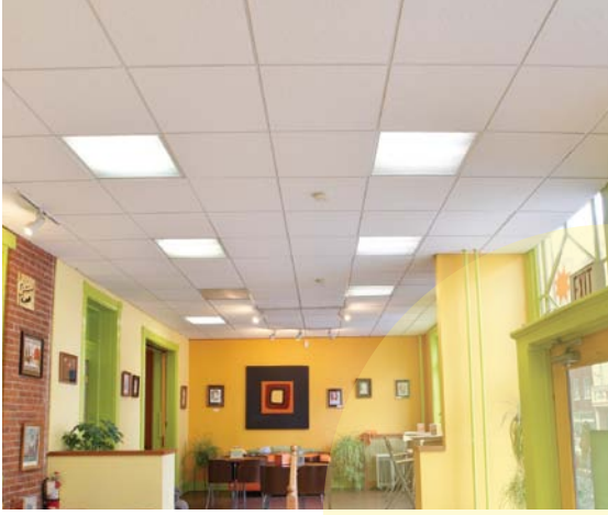
Before: Acoustical tile
